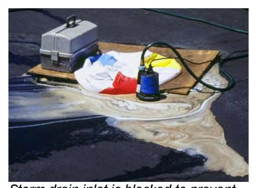
Storm drain inlet is blocked to prevent prohibited discharge. The water must be pumped and disposed of properly.
