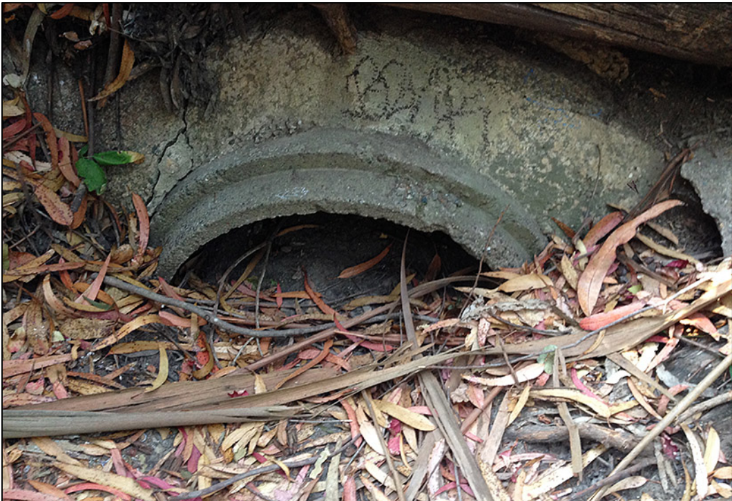
Photograph 12. Looking south at the nearly clogged outflow of the 30-inch concrete pipe that carries flows from the roadside drainage ditch to Whitehouse Creek.
