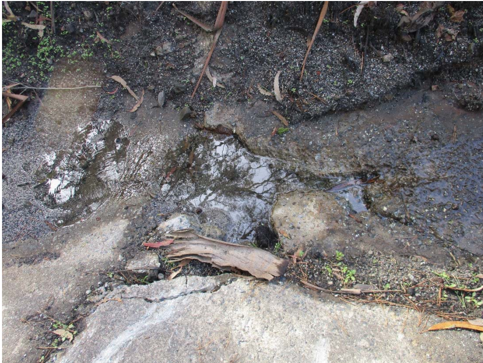
Damaged concrete lined ditch, between Rossi Road and Whitehouse Canyon Road.
