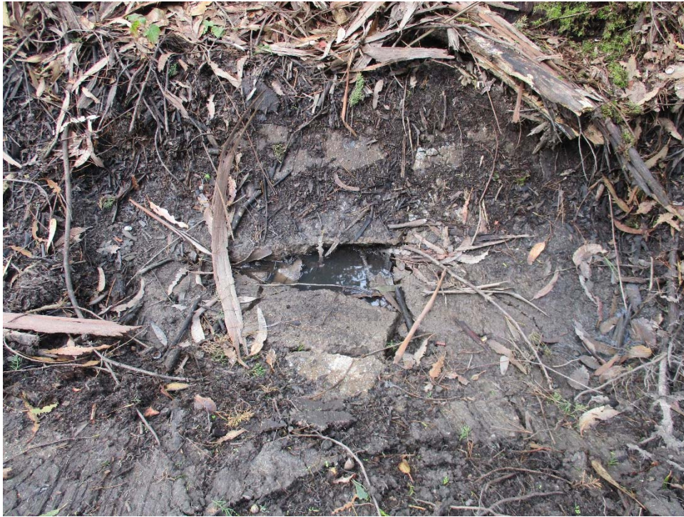
Damaged concrete lined ditch, view southwest towards State Route1.
