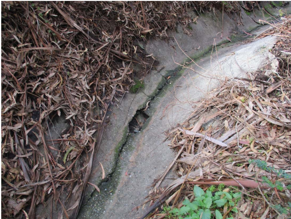
Damaged concrete lined ditch, view west towards State Route 1.
