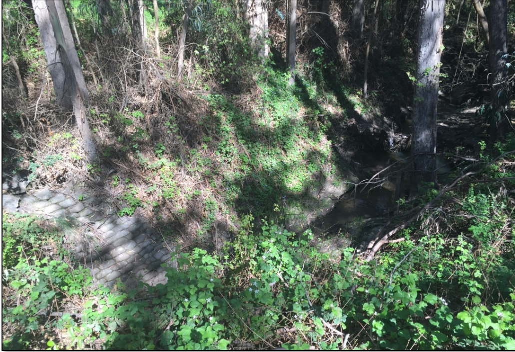
Photograph 9. Whitehouse Creek, looking upstream and northeast at the approximate location of the headwall; showing slope-stabilizing sacked concrete lining the north bank where flows from the 30-inch concrete culvert are directed into Whitehouse Creek.
