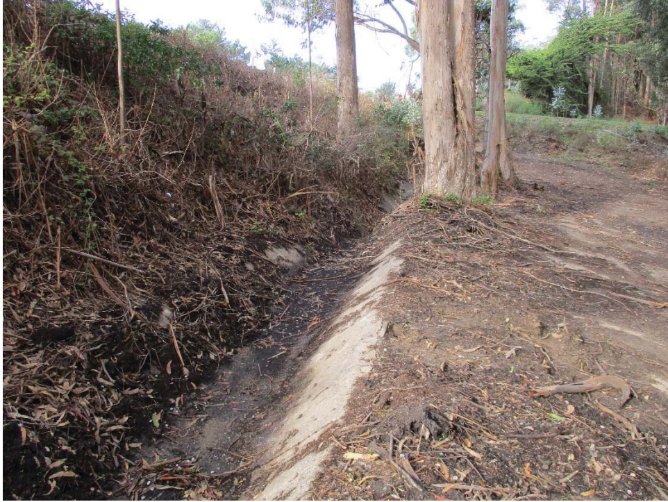
Damaged concrete lined ditch, view northwest towards Rossi Road.
