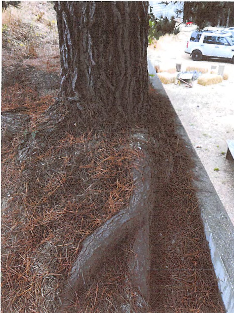
Root system of Tree # 4 on top of retaining wall.
